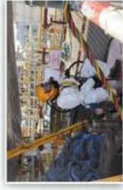
Comprehensive Catalyst Handling and Reactor Maintenance Services
